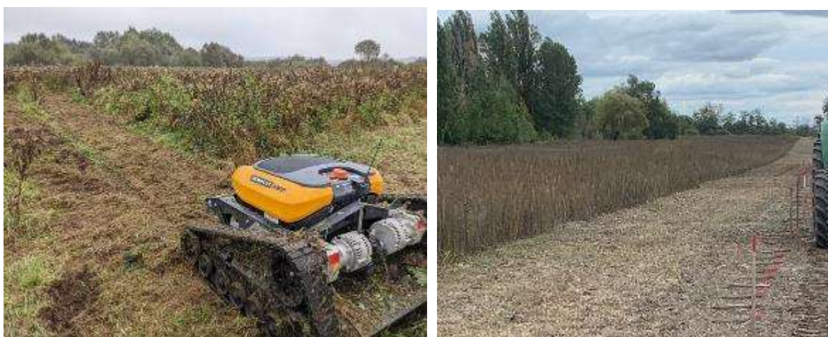
a) Remote-controlled vegetation cutter being demonstrated in a training area b) Long line of vegetation cut by an offset bush cutter, mounted on a tractor
