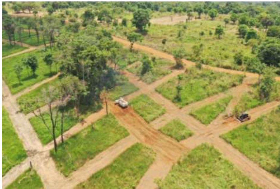
Figure 17 – Ground preparation of systematic technical survey lanes using a bespoke demining machine with tiller attachment – Norwegian Peoples Aid
