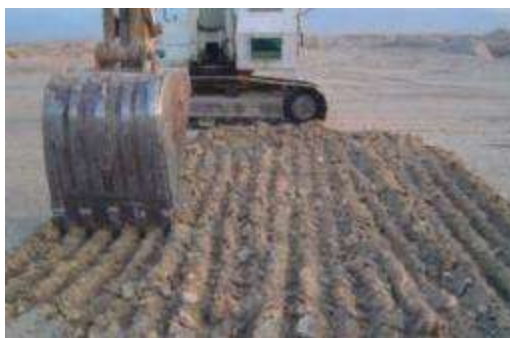
Figure 19 – Tracked excavator with general purpose bucket, breaking up hard ground –The HALO Trust
