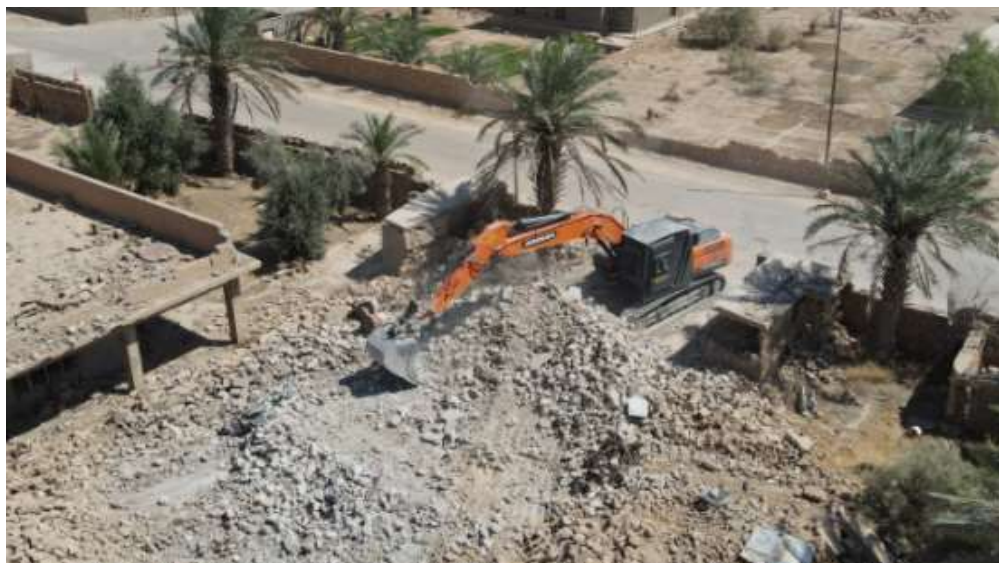
Figure 20 – Tracked excavator with general purpose bucket being used to move rubble to facilitate manual demining – Norwegian Peoples Aid
