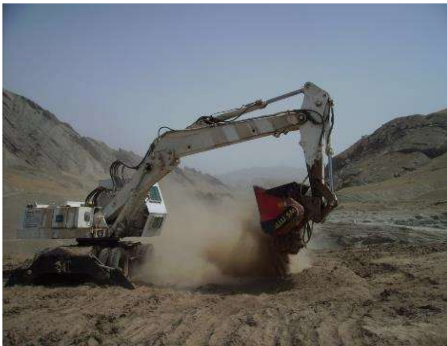
Figure 2 – Crushing bucket attached to a wheeled excavator, processing material from a spoil pile – The HALO Trust
